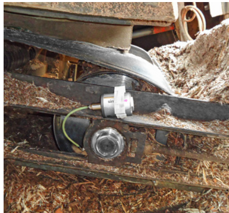
The Yball-bearing unit of a conveyor belt is continuously supplied with lubricant.
