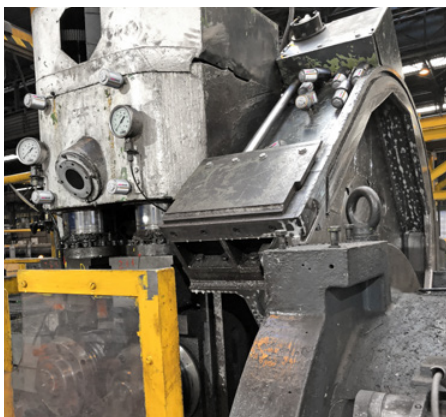
Several simalube lubricators and IMPULSE lubricate the columns (left) and the drive unit (right) of the nibbling machine.
