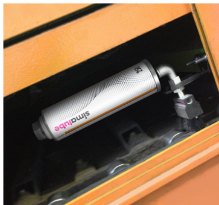
The conveyor belt chain in a recycling factory is automatically lubricated and cleaned with simalube and brush.
